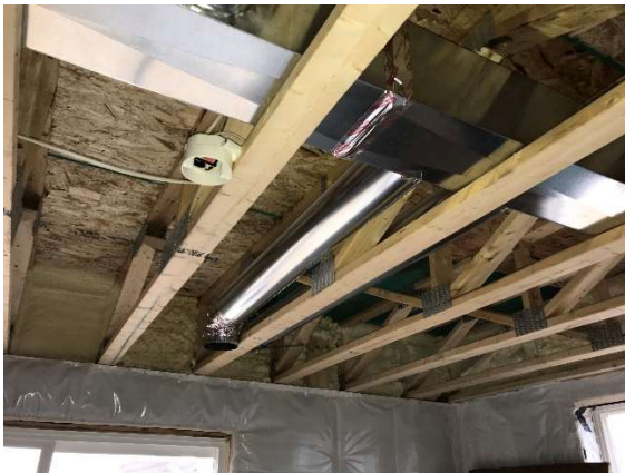
9. Ducted and sealed supply air
