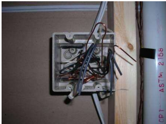
1. Electrical rough-in have all boxes made up and ready with minimum 6-inch tails.
