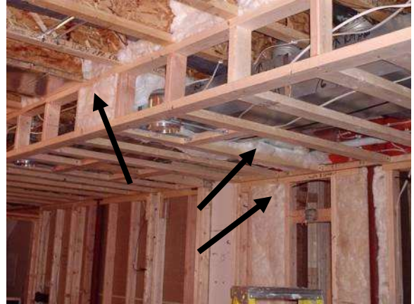
6. Fiberglass insulation used as fire-blocking every 10 feet horizontally in the soffit and separating soffit from wall cavity.
