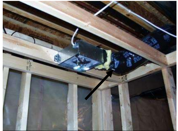
8. Insulated flex duct from bath fan leading to exterior, minimum 3 feet from exterior wall in required to be insulated.
