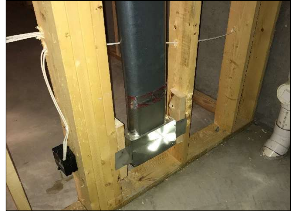
10. Ducted and sealed return air.
